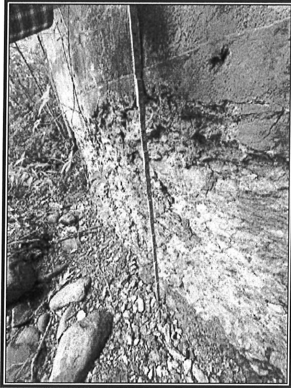
Photo 9: Concrete loss up to 6 inches.
