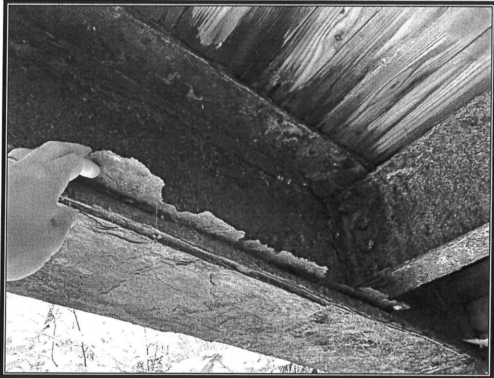
Photo 3: Steel stringer with significant section loss.
