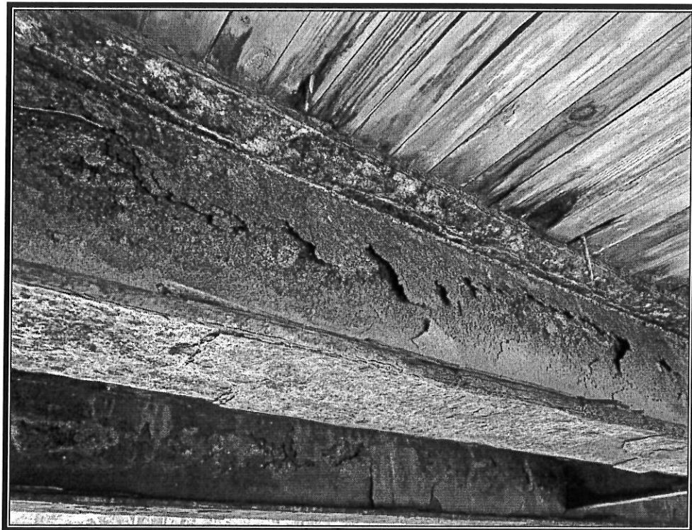
Photo 4: Steel stringer with significant section loss.
