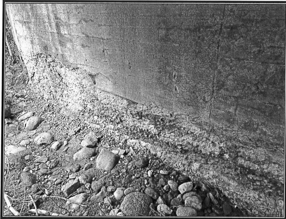
Photo 8: Eroded concrete due to freeze thaw at waterline.
