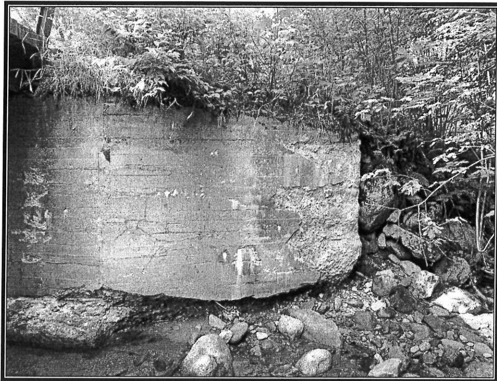
Photo 10: Undermined abutment and wingwall.
